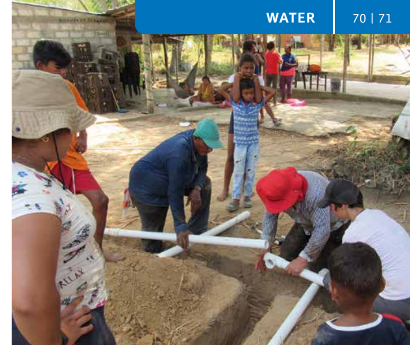
New pipes are installed as part of the rehabilitation of the drinking water supply.
