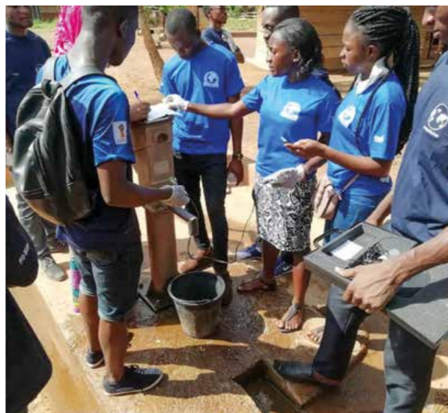
Committed students from Germany and Ghana work together in a well construction project in the Brong-Ahafo region.
