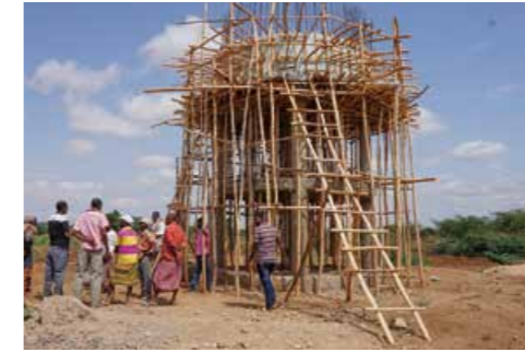
Ultrafiltration technology and a water tower have helped to improve the situation of the people of Adadle woreda.
